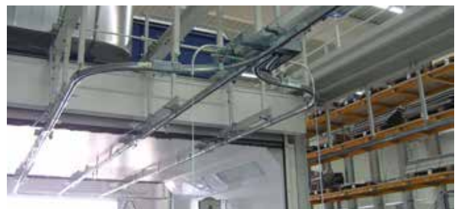
Overhead handling system
